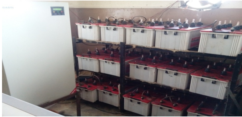
Photo: Battery Backup
