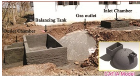
Fig 7.1 Biogas plant installed in the campus
