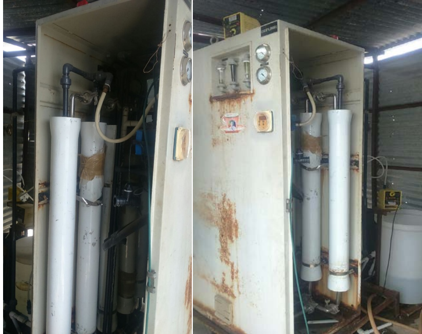
Photo: Two RO Unit at Boys' Hostel
