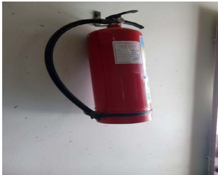
Photo: Fire extinguisher
